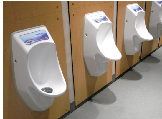
URIMAT Waterless Urinals as specified by McDonald's Restaurants Ltd
